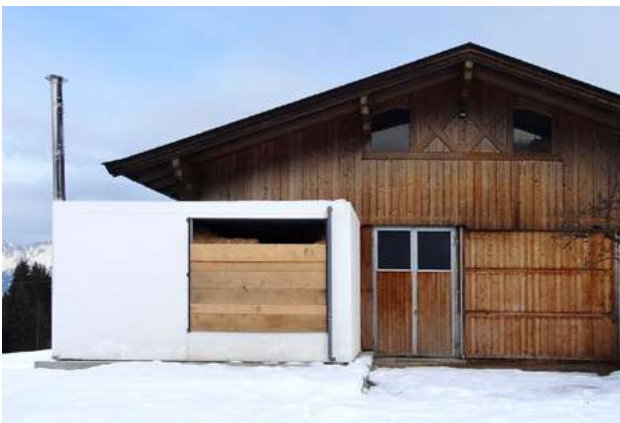
Single floor heating module 35 kW wood chips, farm
